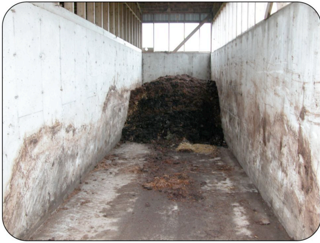
Figure 4. These concrete walls are 2.4 m high (8 ft) but the compost is never piled deeper than 1.8 m (6 ft). If building again, the operator would have made the bin 0.6 m (2 ft) wider than his loader, as it is a tight fit in a long, narrow bin like this.
