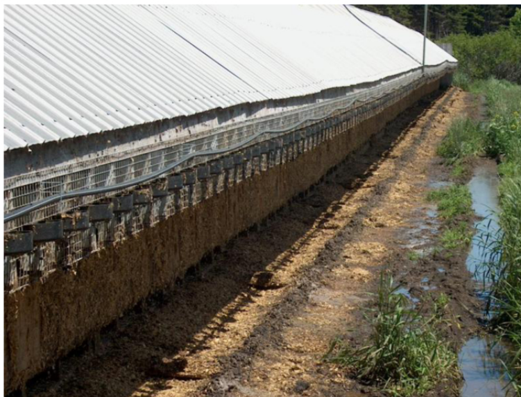
Poor drainage around shed which creates ideal fly breeding area.
