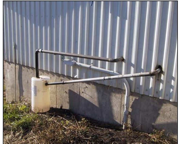
Figure 2: Collection system for two vacuum pumps
